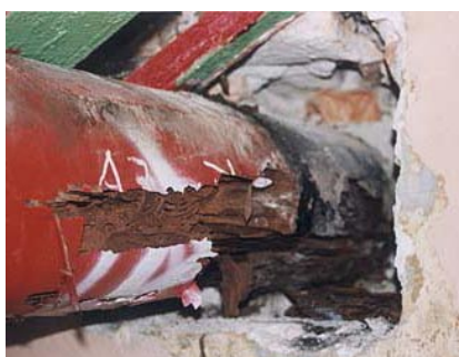
Decayed Beam End
